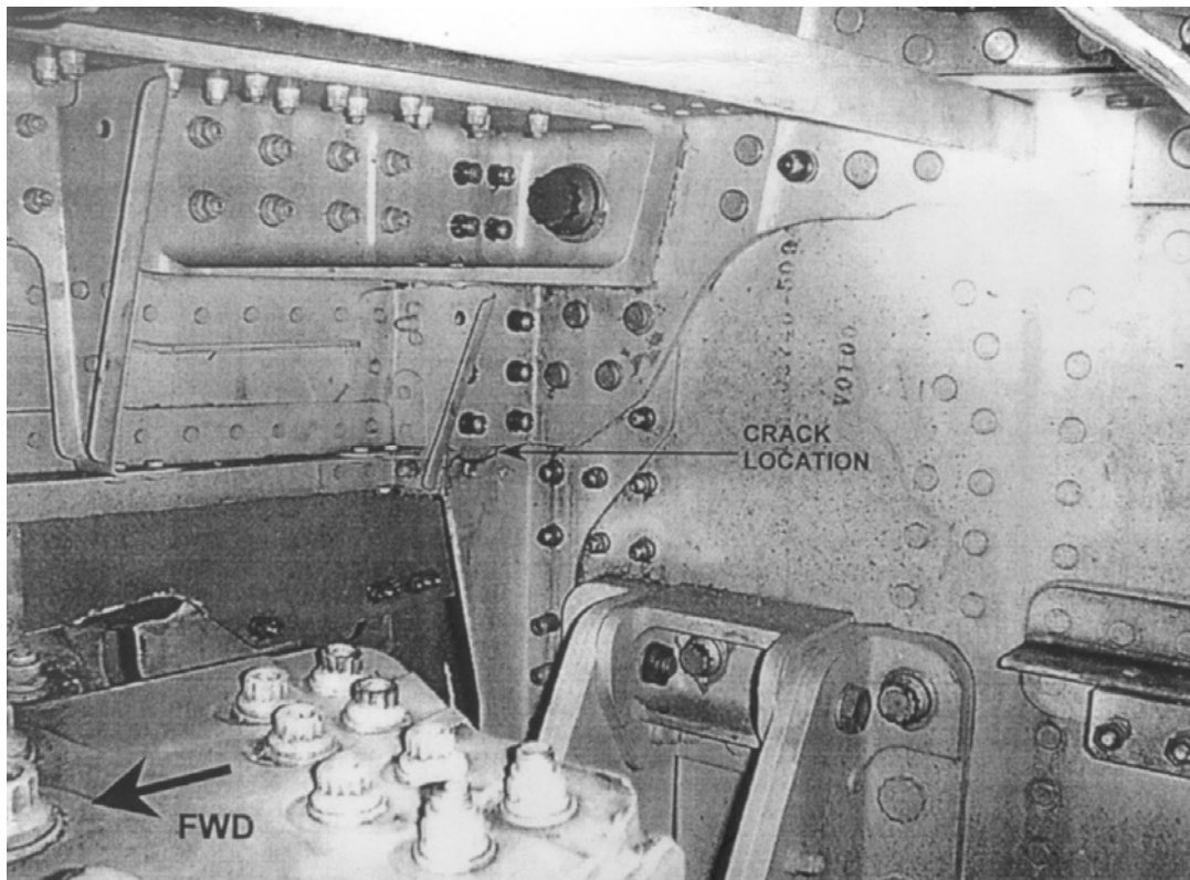
Figure 3: Fatigue crack in an Ansett B767 Body Station 1809.5 bulkhead outer chord
