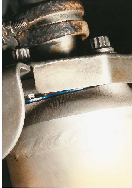
Figure 5: CF6 Gap at Leaking Flange
